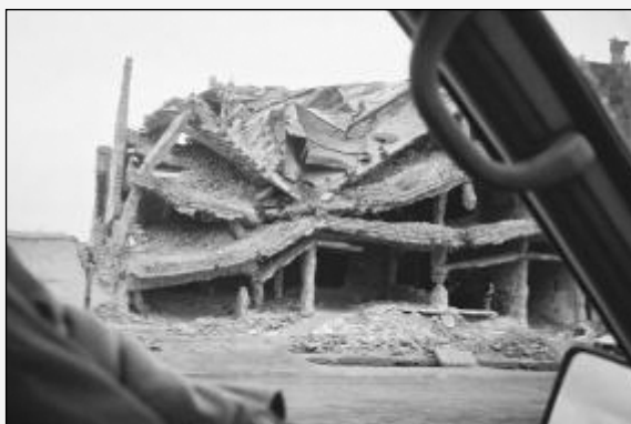
Figure 1 A war damaged building in Kabul: a graphic image of the current state of Afghanistan. Visionary politicians are exploring ways in which a sustainable minerals approach can help restore a peacetime economy and government.
