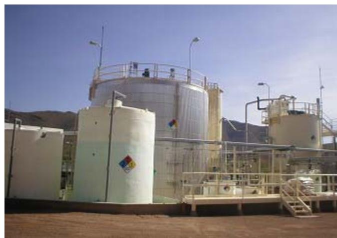
Figure 6: BioteQ plant, Bisbee mining district Arizona
